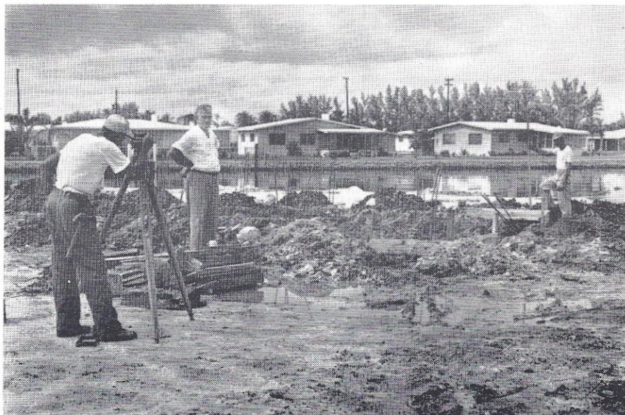
Lot surveying was the first step in the many phases of construction that went into the completion of your Lauderdale Harbors home. The above picture shows William Hopkins, left, layout foreman, using a transit and setting levels as Al Clark, center, building superintendent, looks on.
