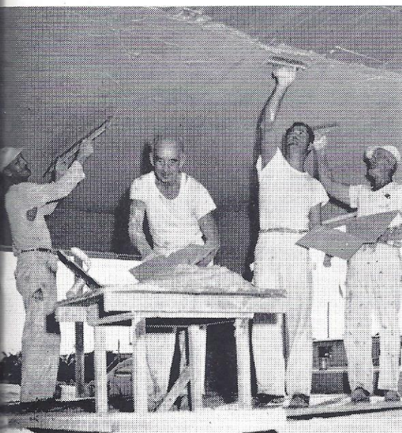
Plasterers are shown applying a rough coat of plaster over the rock lathing. A smooth white finish coat followed.
